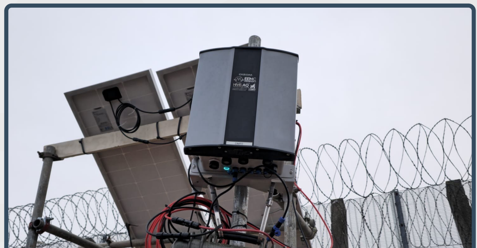
INSTALLATION DETAILS 2 Units of Oizom Air Quality Monitors
